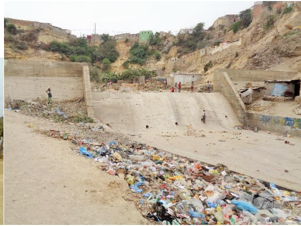
The area affected by the flood in Lobito
